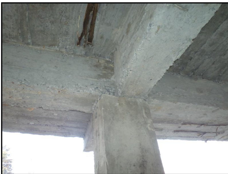
Figure 28: Wrong Practice of Beam Column Junction
