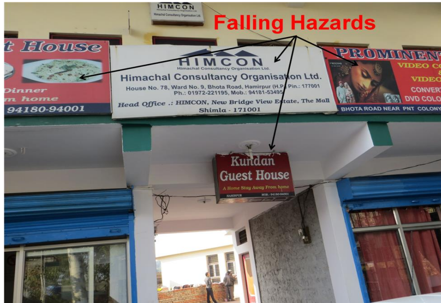
Figure 41: Falling hazards in a building
